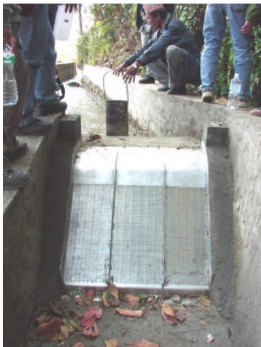
Figure 4.1 Coanda screen at forebay of Cha Khola MHP
